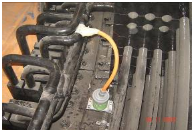
Figure 2: Coupling capacitors at phase insulated bus bars
