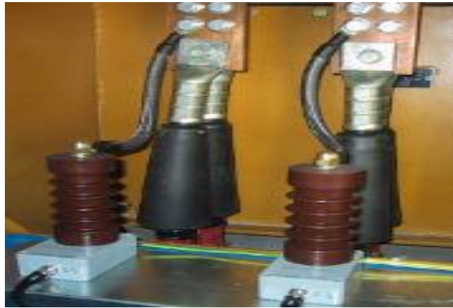
Figure 3: Coupling capacitors direct at the generator high voltage terminals
