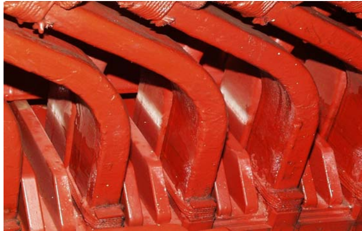
Figure 1: Example of a PD (at the white bands) occurring due to deterioration of the slot conductive coatings and/or the silicon carbide stress relief coatings.
